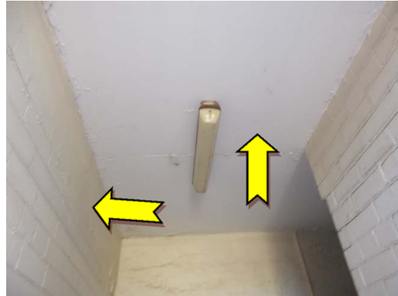
Photo 2. Interior, men's toilet, ceiling and walls – suspected lead-containing upper white and cream coloured paint systems.
