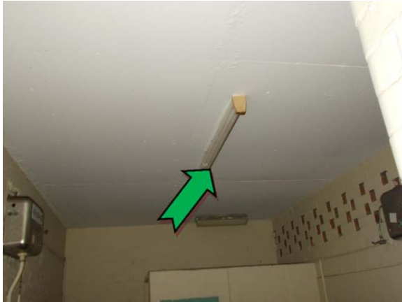
Photo 1. Interior, men's toilet, single tube fluorescent light fitting – suspected non PCB-containing capacitor.
